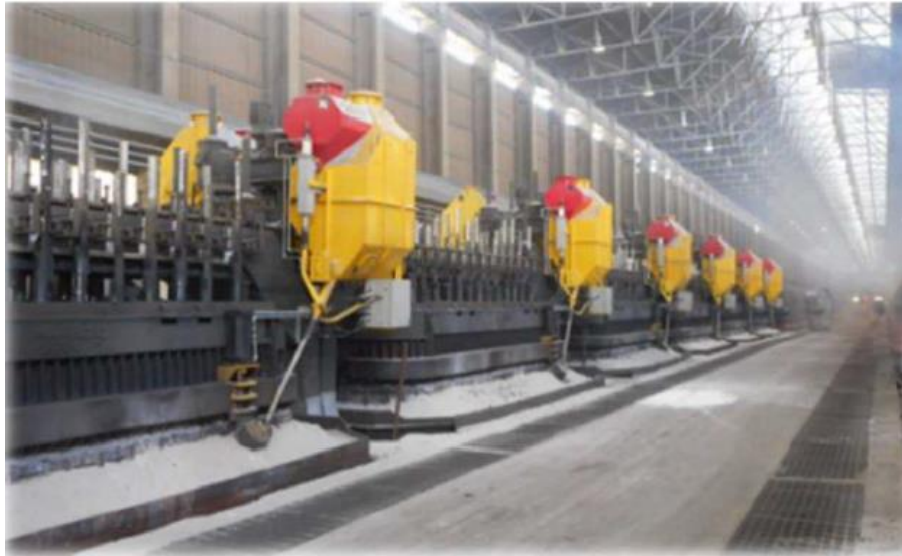
Figure 10. Point feeder at CBA Söderberg cells, alumina duct, and feeding chute [5].
